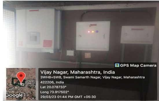
Figure 15. Installed Solar Charge controller
