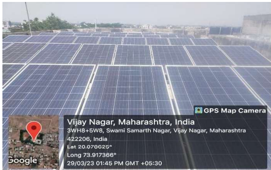
Figure 14. Installed Solar Panels
