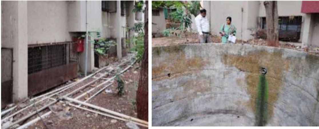
Figure 5 Rainwater harvesting well with pipe discharging water
